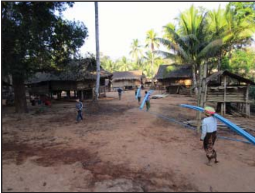
Tubing is placed throughout the village to bring clean water to all
