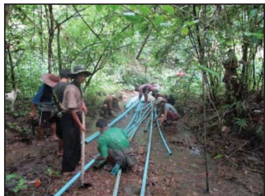
Laying pipes through the jungle to bring clean water to the village
