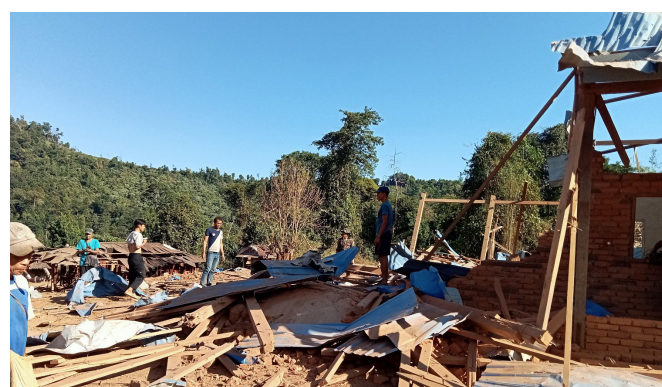
Figure 14. A middle school destroyed by an air strike
